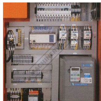
Electrical Control Cabinet
