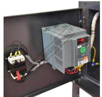
Schneider Inverter Control
