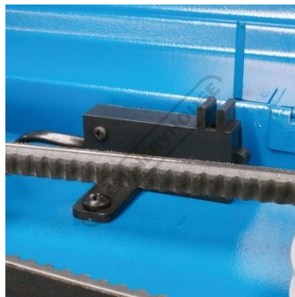
Safety Micro Switch on Pulley Guard
