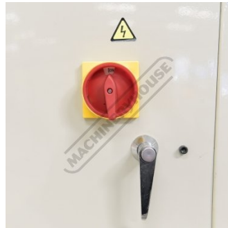
Main Isolation Switch
