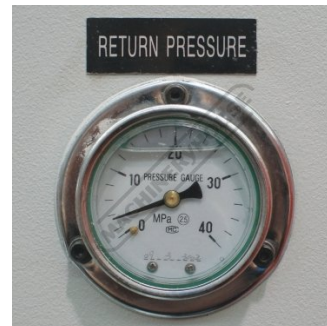
Return Pressure Gauge
